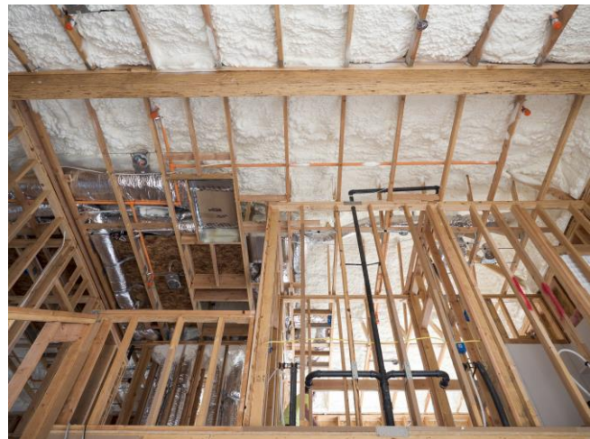
Open-cell spray foam installed below roof deck
