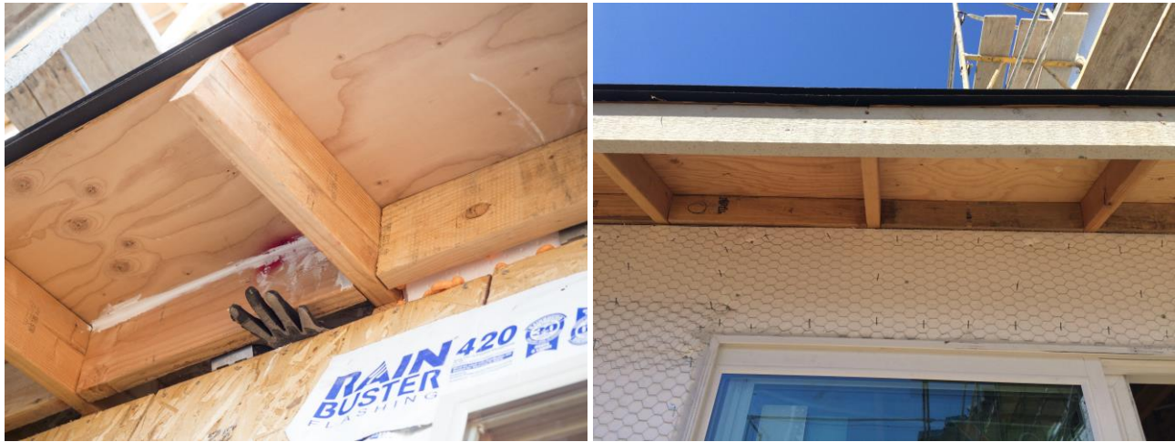
Figure 7. Gap at eaves requiring manual blocking prior to AeroBarrier (left), example of exterior ridged foam used to close the gap prior to open-cell spray foam installation (right)
