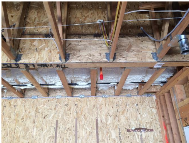
Open-cell spray foam installed at rim joist Figure 3. Photos of homes sealed under Option 1
