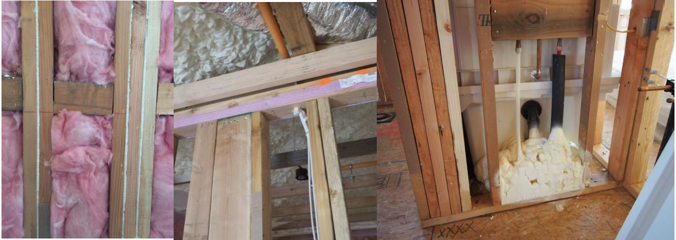
Can foam used between double studs Foam gasket to seal drywall between house and attic Spray foam used at plumbing penetrations
