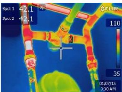
Thermal Image of water and space heating piping in a resident unit (red = heat escaping)
