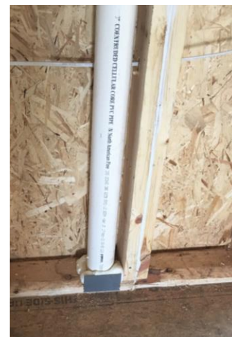
Plumbing penetration and caulk gap between studs
