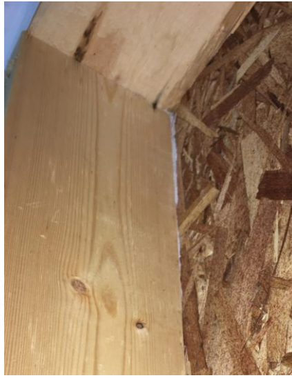
Gap between framing and sheathing
