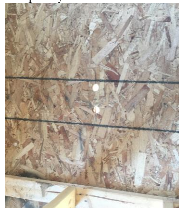
Tape used to temporarily seal 1" holes in flooring
