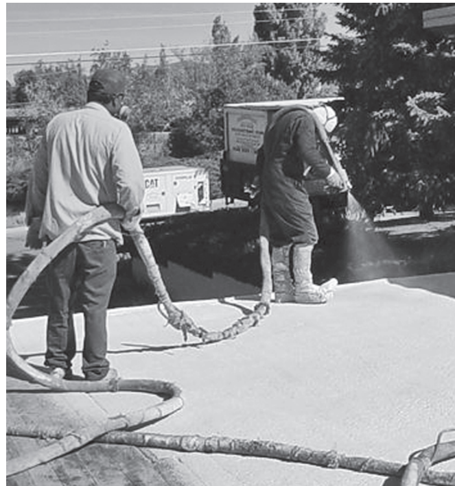
Figure 2. Spray polyurethane foam roofing can only be installed when the weather is warm, dry, and relatively windless. [Photo credit: Goodrich Roofing Co.]
